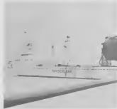
Huge 575-ton vacuum tower brought in by the Netherlands' field office was set in place.
